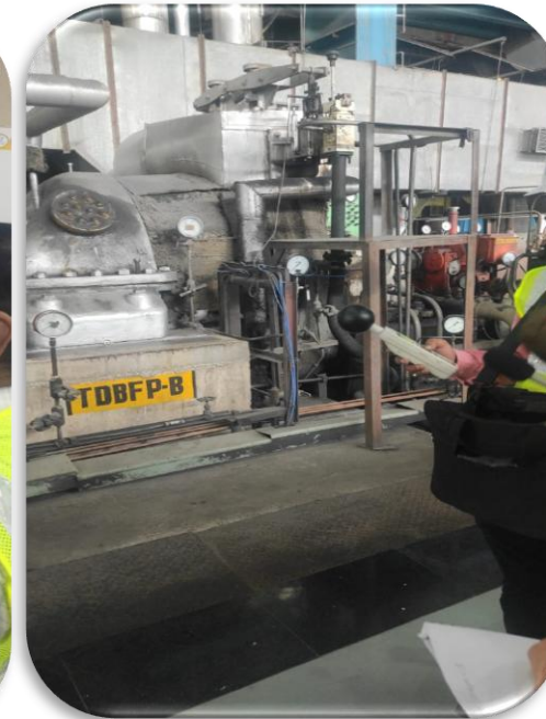
Light, Noise, Heat measurement at TG & Boiler area measurement
